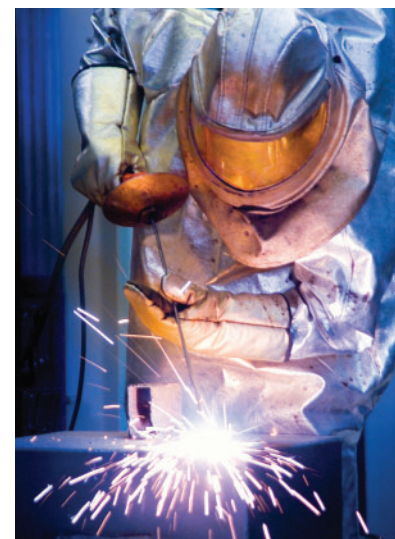
Figure 1 A worker in heat-resistant protective clothing uses an oxyacetylene torch to cut steel.
